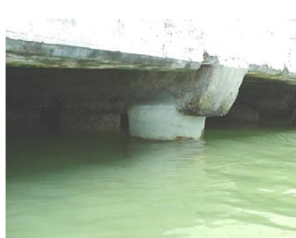
View of the rehabilitation with Subcom T.260 replacing concrete between piles and platform
