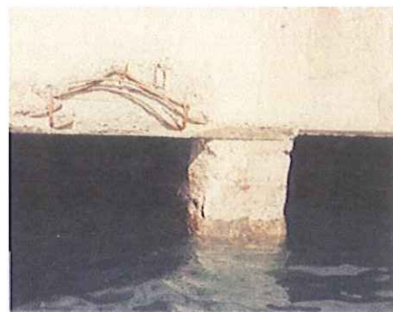
Coping beam heavily damaged with exposed re-bars.
