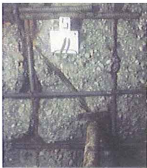
Submerged coping beams area after sandblasting evidencing exposed re-bars.
